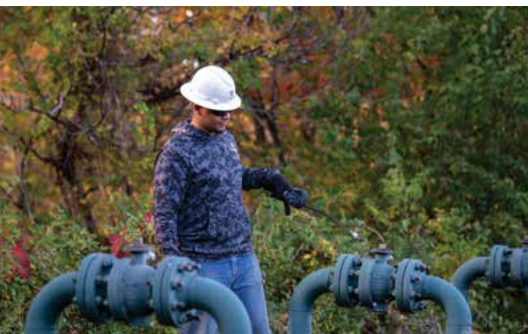
Diversified's suite of handheld emissions technologies include the Teledyne FLIR GT-44. Well tenders survey wells across the company's operating areas.
