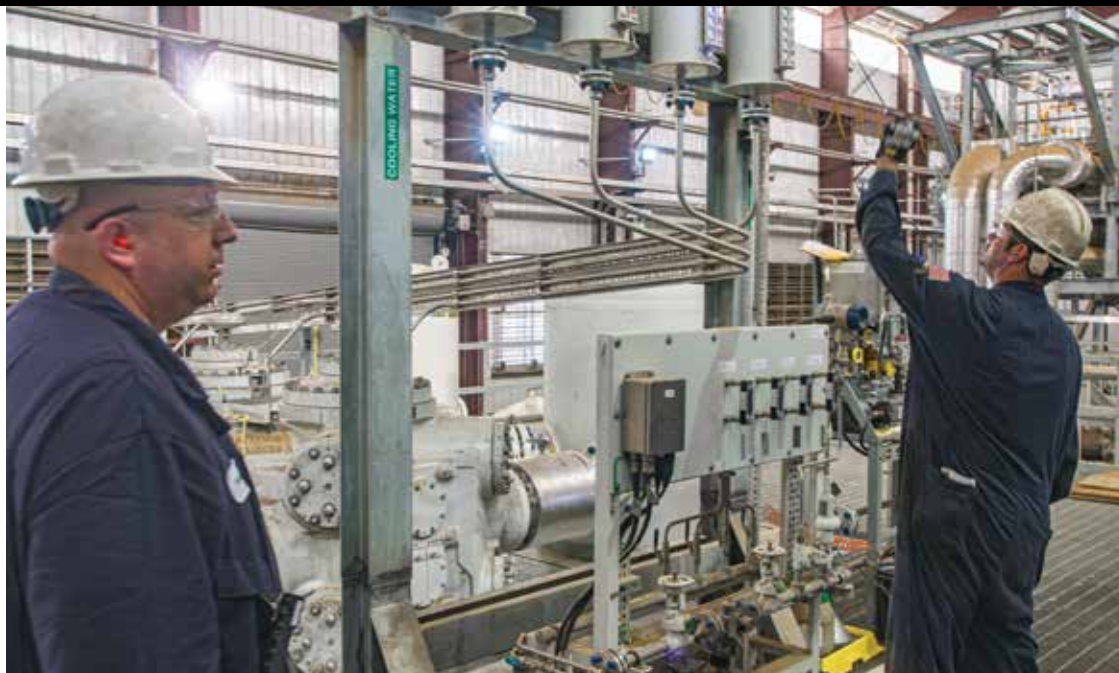
Damon Knupp and Torrey Ollermann (left) check the oil level of the sight glass in a compressor building at the Tioga gas plant.
