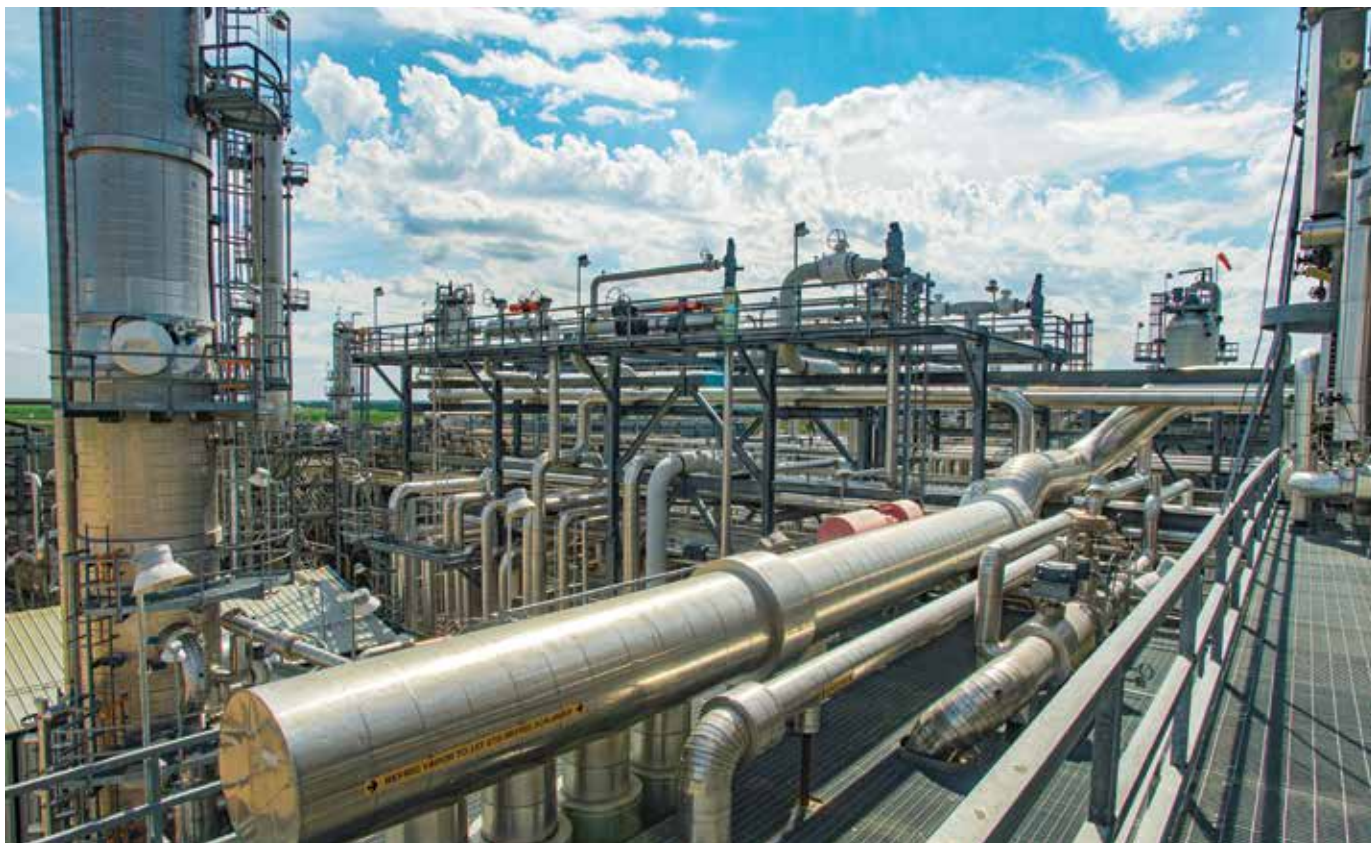
Pictured above, the refrigeration process equipment at Hess' 250-MMcf/d Tioga gas plant in Tioga, N.D.
