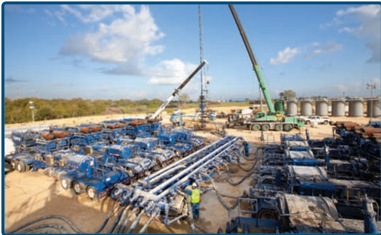
Schlumberger performs a HiWAY fracture stimulation job on one of BHP Billiton's Eagle Ford wells. (Photo courtesy of BHP Billiton)
