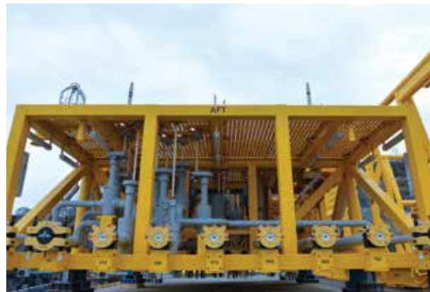
The Gullfaks subsea wet gas compressor
