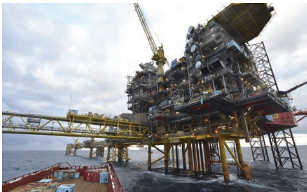
The redevelopment plan includes a new processing platform and a new accommodation platform for Tyra East (shown here) and Tyra West. (Source: Maersk Oil)
