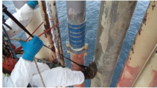
Composites have been used for offshore repairs for years in a broad range of applications, such as riser pipe sections close to the water line and longer pipe networks that are hard to get to. Here, trained technicians use rope access to repair a riser. (Source: Clock Spring)
