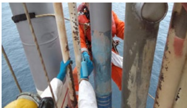
Using rollers to apply adhesive, the installation team places and secures the composite sleeves. (Source: Clock Spring)
