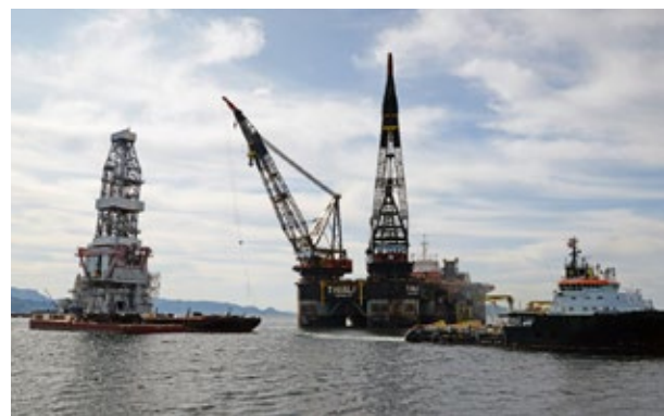
The assembly operation of the Johan Sverdrup drilling platform takes place in Klosterfjorden near Stord in Norway. (Source: Arne Reidar Mortensen/Statoil)
