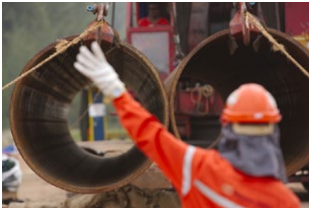
A worker helps unload pipes for the Ichthys LNG project. (Source: Inpex)
