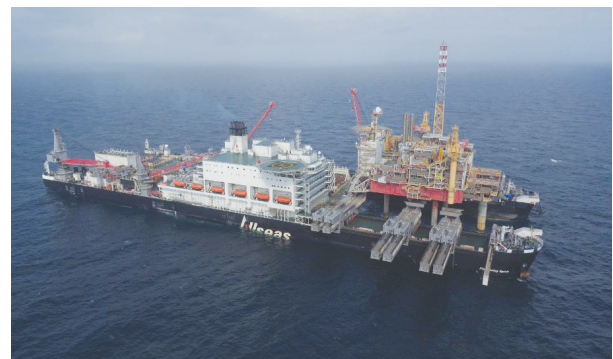
The Pioneering Spirit straddles its twin bows around the Yme platform before securing the structure, cutting the jackup facility's steel legs and lifting the 13,500-tonne topsides. (Source: Allseas)
