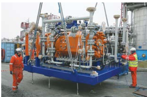
The Åsgard subsea compressor is installed at the K-lab test facility in Kårstø north of Stavanger. (Source: Statoil)
