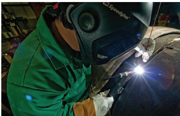
Exterior weld of low pressure housing of a subsea wellhead. (Source: GE Oil & Gas)
