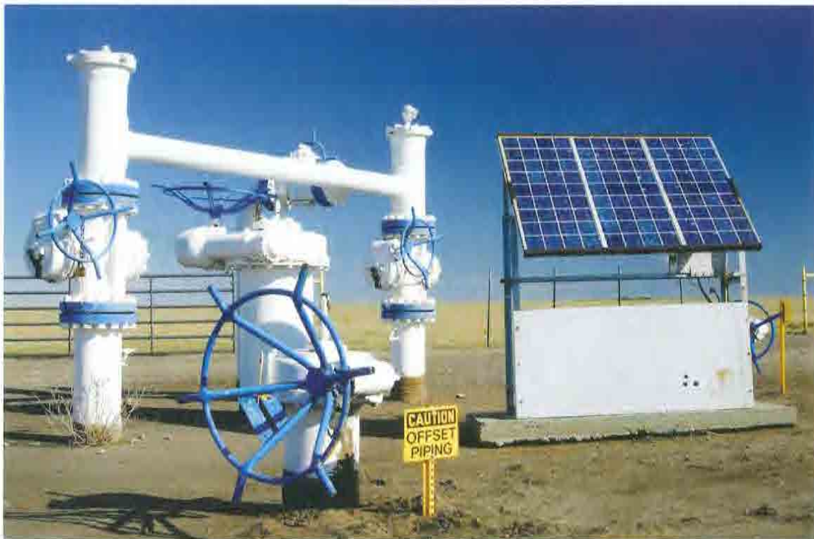
Solar panels provide electric power for monitoring equipment on a pipeline in Texas.
