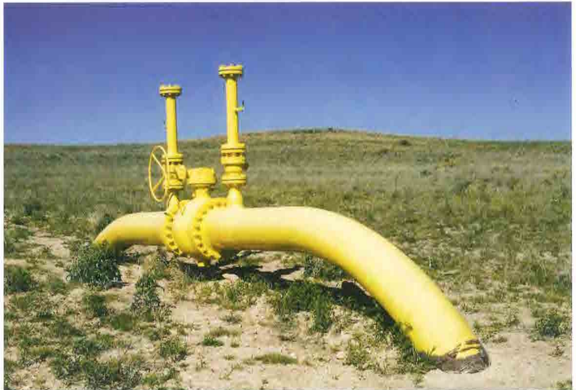
A petroleum pipeline traverses Texas, home to a majority of the midstream systems that support Permian Basin production.
