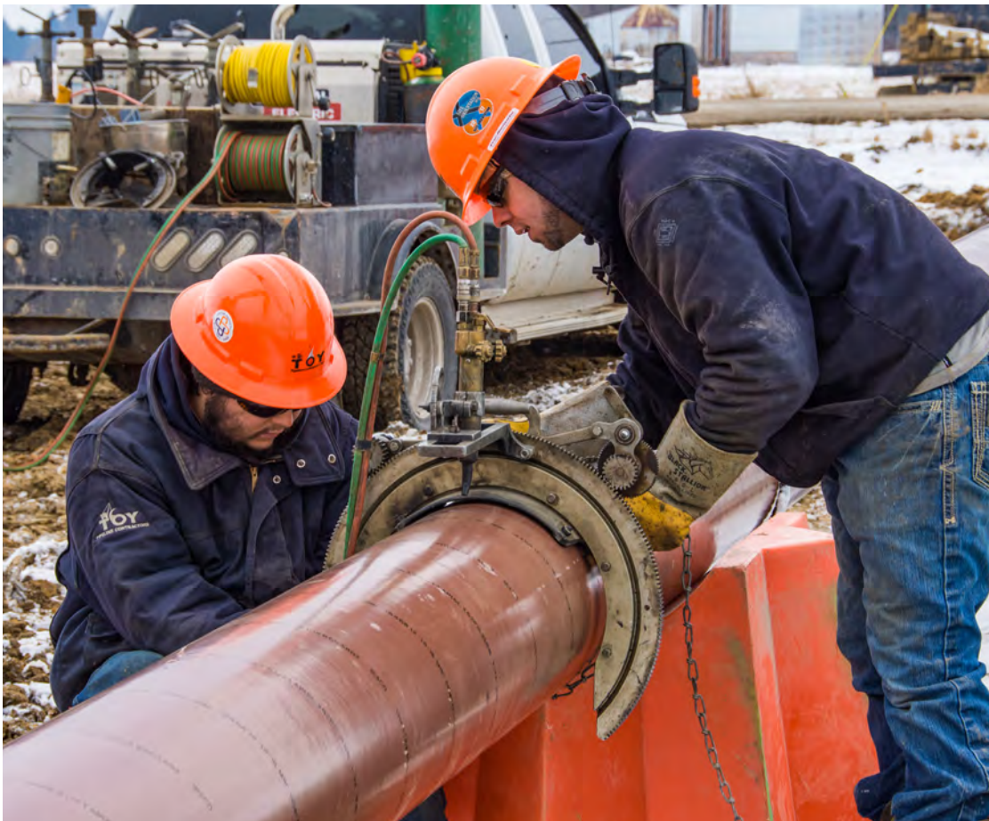
Pipeline contractors beveling pipe and preparing to make a weld. Facing page, a driller directing his crew during a connection.
