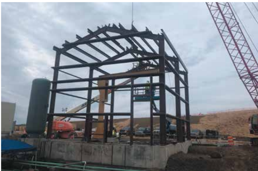
The housing for an Atlantic Sunrise compressor station goes up on the right-of-way in Wyoming County, Pa.
