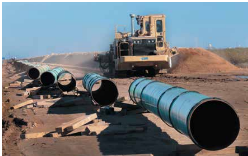
This will need to be a common Permian scene in coming months as midstream players race to add capacity. This pipe went into one spread of ONEOK’s Roadrunner Gas Transmission system that moves Permian gas south to Mexico. Source: ONEOK Inc.
