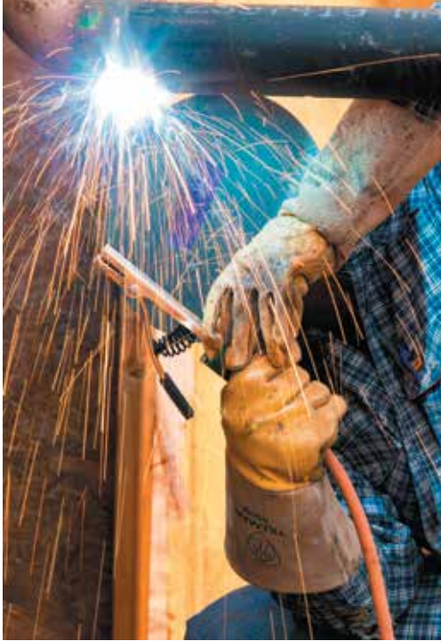
Surging Midcontinent production could spark major additions to Oklahoma's midstream infrastructure. This welder lays a bead on a pipe inside an EnLink plant in the Sooner State. Source: EnLink Energy Partners LLC
