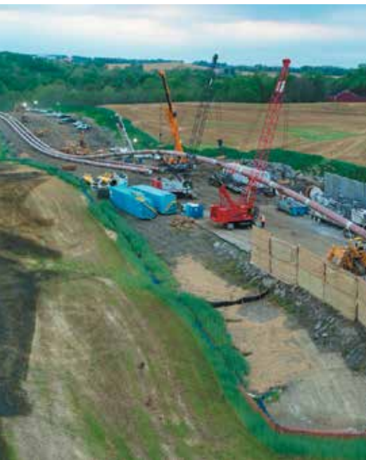
Crews ready pipe to go under the Conestoga River following a directional drilling job under the stream.
