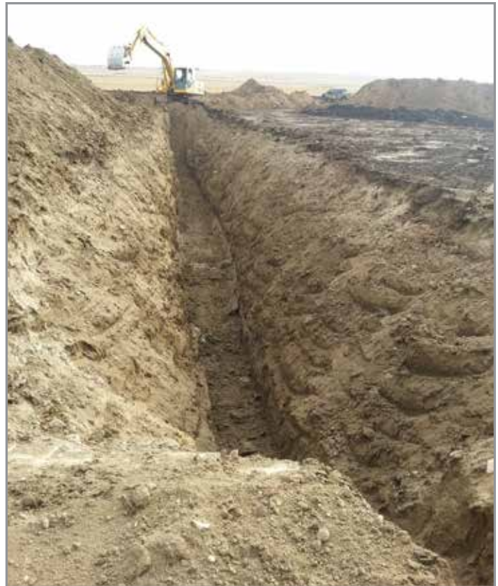
Cleanup Efforts | In an effort to recover released material after the leak, interception trenches are dug to collect oil from saturated soils in the shallow subsurface. (Courtesy: Tesoro)
