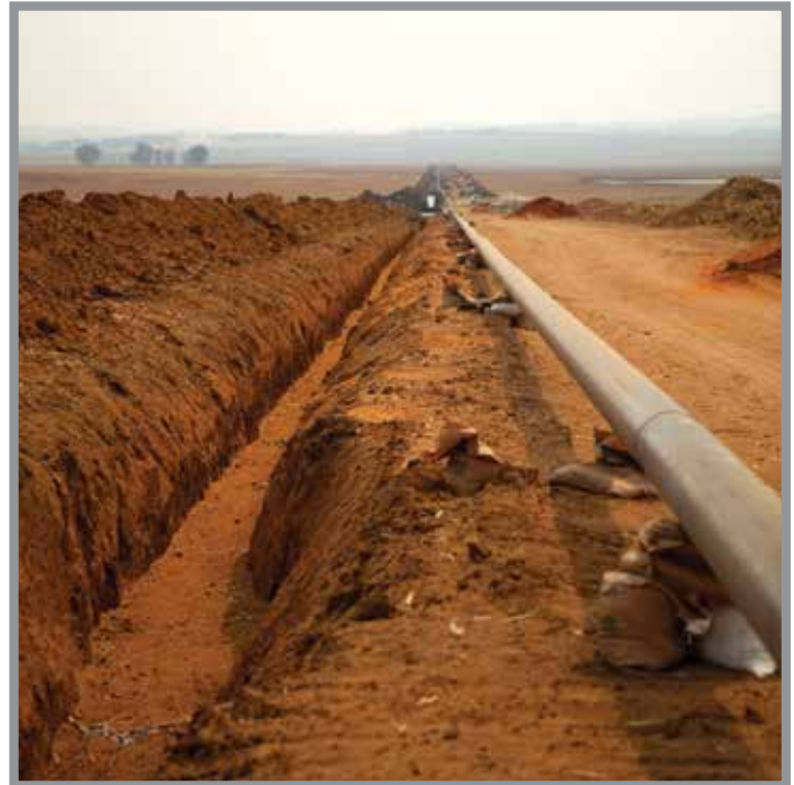
Operations Under Way | The Pecos River Pipeline began operations after completing Phase I of its construction.
