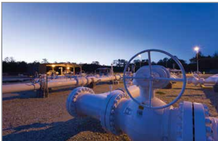
A one-third interest in the Southern Hills Pipeline was included in a $1.15 billion dropdown deal between DCP Midstream Partners and its GP, DCP Midstream LLC. The Lockwood Pump Station in Humble, Texas, pictured above, helps this system achieve a capacity of 175,000 bbl/d. (Source: DCP Midstream)
