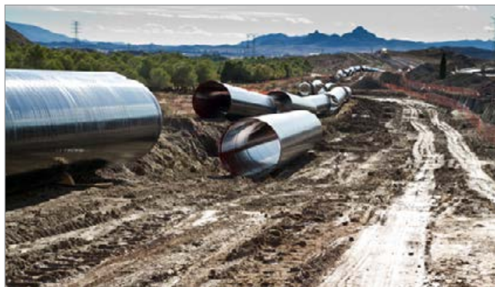
CLEARED | Alliance Pipeline's Tioga Lateral Pipeline project in North Dakota received FERC approval.
