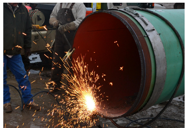
Hypertherm Powermax plasma systems are now being used on the Ruby Pipeline (Photo courtesy: Hypertherm Powermax).
