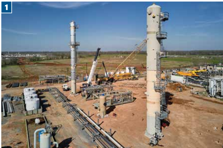
1. Aerial view of Clearfork's newly installed 108-inch diameter amine contactor tower at its Holly 6 amine treating facility in northeast Red River Parish, La. (facing west).
